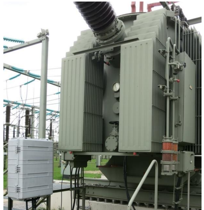
Fig 5 Measurement system at transformer
